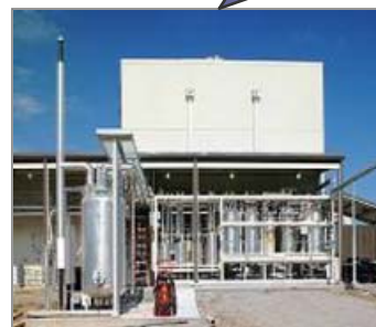
Refining Pilot Unit 2 BPD
