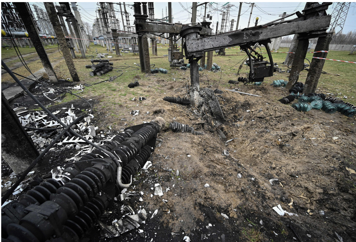
Damaged equipment at a high-voltage substation of the operator Ukrenergo after a missile attack in central Ukraine on November 10, 2022.
