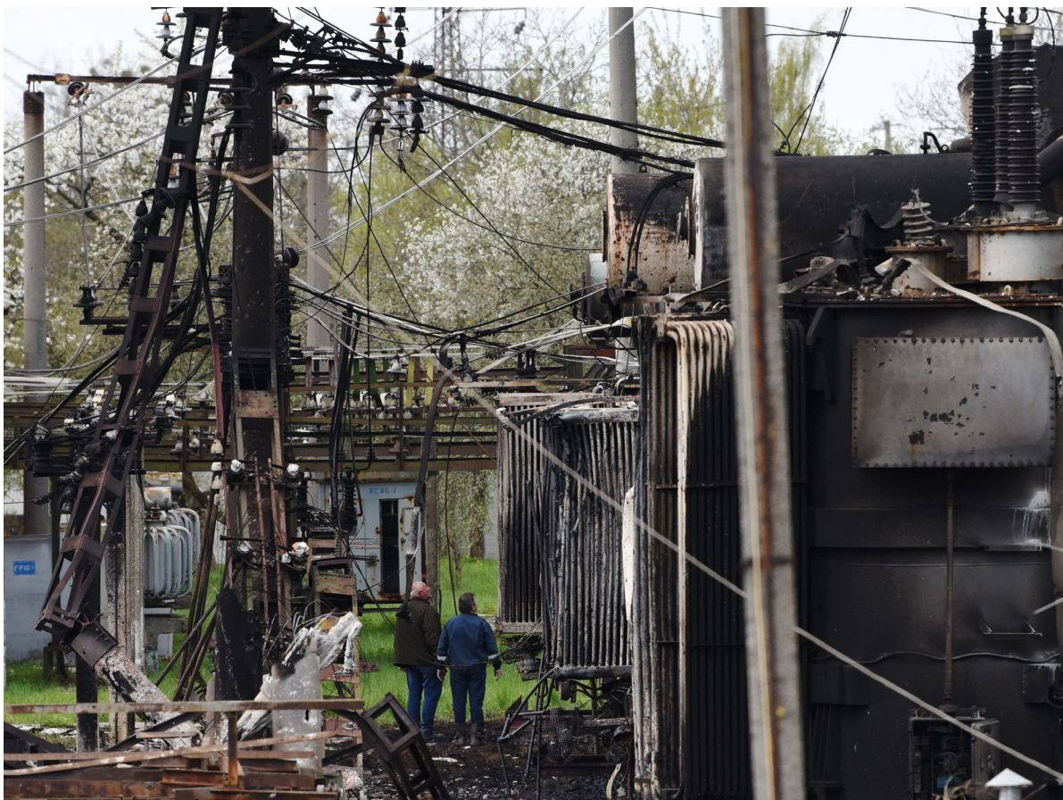
Workers look at a power substation damaged following a missile strike in the western Ukrainian city of Lviv on May 4, 2022, as Russia’s defense ministry said that its air- and sea-based weapons have destroyed six electrical substations near railways, including around Lviv.
